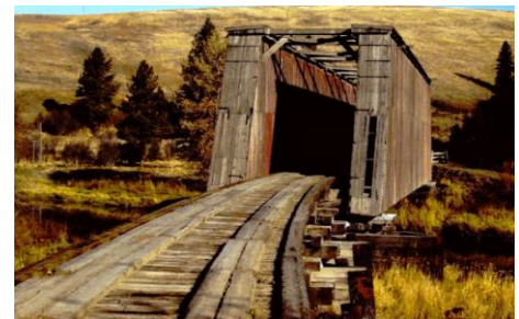
Colfax Bridge, Whitman County, Washington, in 1983. Lost to a wildfire on September 7, 2020
