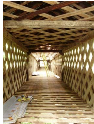
Horton Mill Bridge during repairs, Courtesy Friends of the Covered Bridges of Blount County
