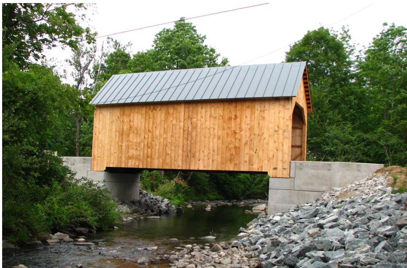
Bower's Bridge (45-14-11) in Windsor County, Vermont After being washed downstream by floodwaters in August 2011 (top) the bridge was repaired and set on new abutments on July 14, 2012 (bottom).
